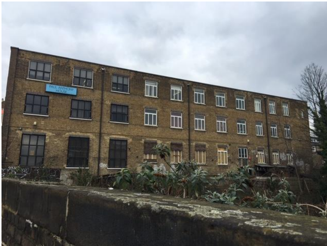
The existing south elevation of 724 Holloway Road as seen from the railway bridge
